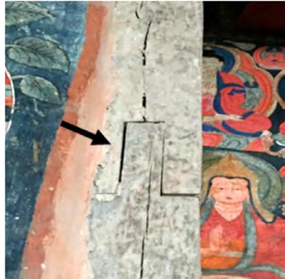
Figure 6 Finger joints in the pillar (arrow).
